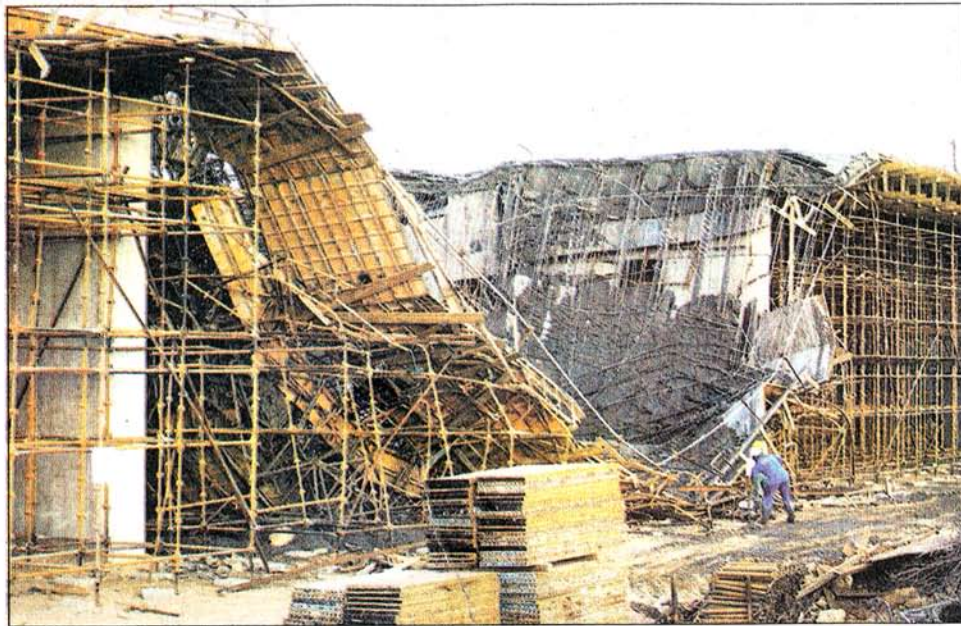
DEADLY LETDOWN: Scenes such as this collapse of Port Elizabeth's Coega Bridge in 2003 are becoming more frequent as unqualified contractors treat the industry as a money-spinner, not a long-term career choice Picture: © THE HERALD
